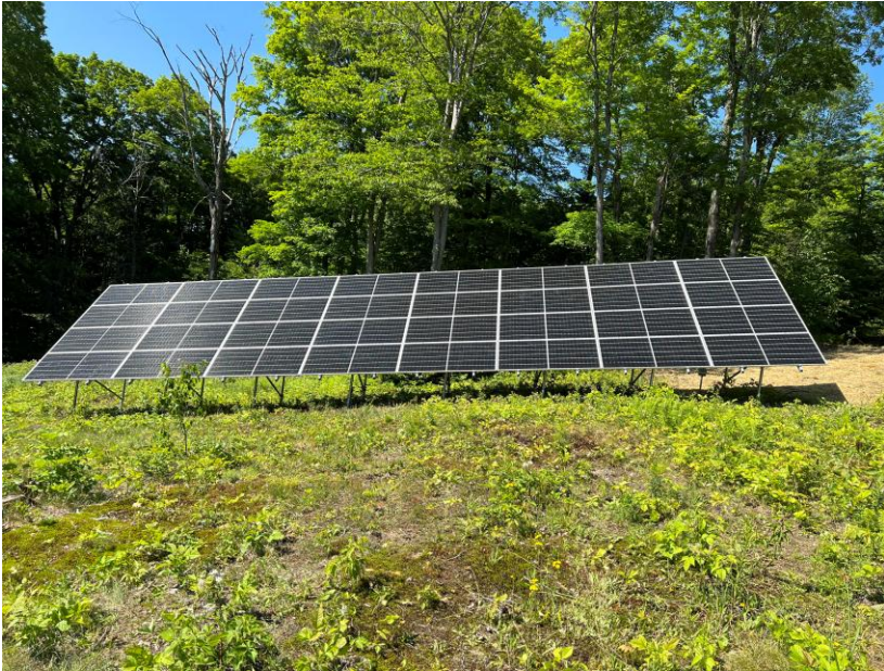
15kW residential solar array in Barnard
