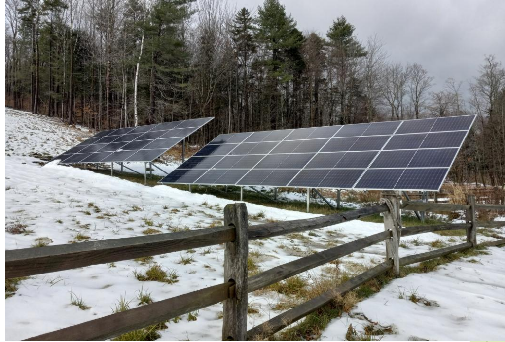
15kW AC residential solar array with 435W panels (66'x12')
