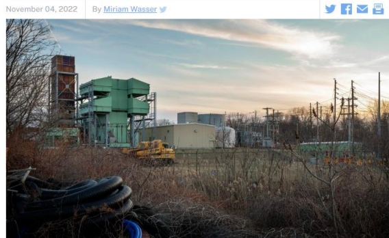
The Peabody Municipal Light Plant's Waters River substation on Pulaski Street currently has two gas peaker power plants. The Massachusetts Municipal Wholesale Electric Company has approval to build a third plant in the flat grassy area where the two yellow trucks are parked. (Robin Lubbock/WBUR)
