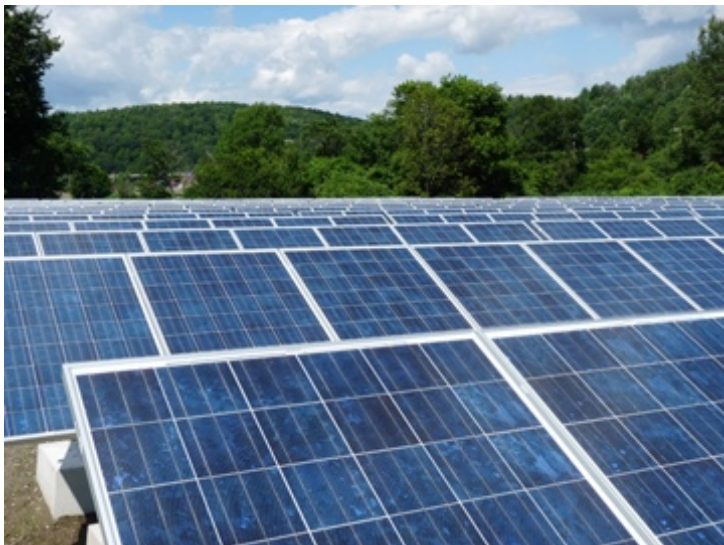
Green Mountain Power's Berlin, VT Solar Facility
