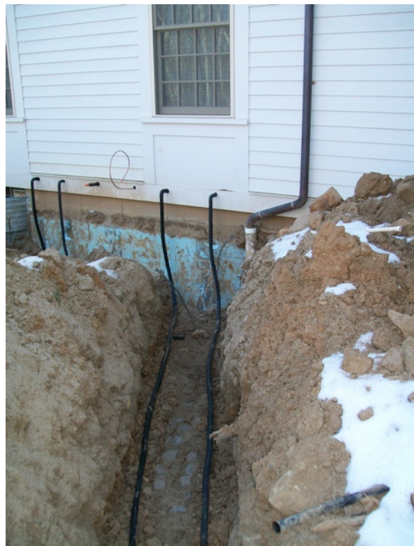
Tubes carrying water in a "closed loop" system ready to be buried in the earth. Water warmed by the earth flows into the house's geothermal heating system, cold water flows back outside to be re-heated.
