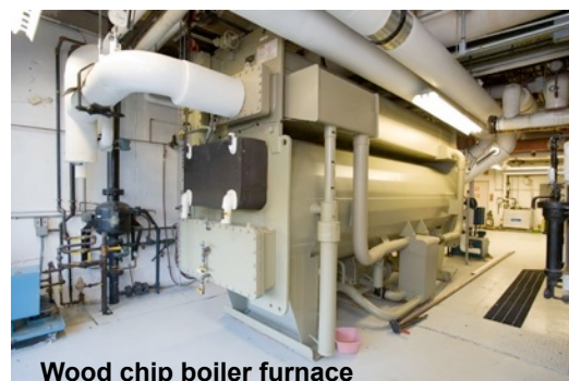
Wood chip boiler furnace
