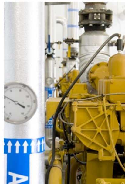
Pipes, equipment, and a biogas power generator
