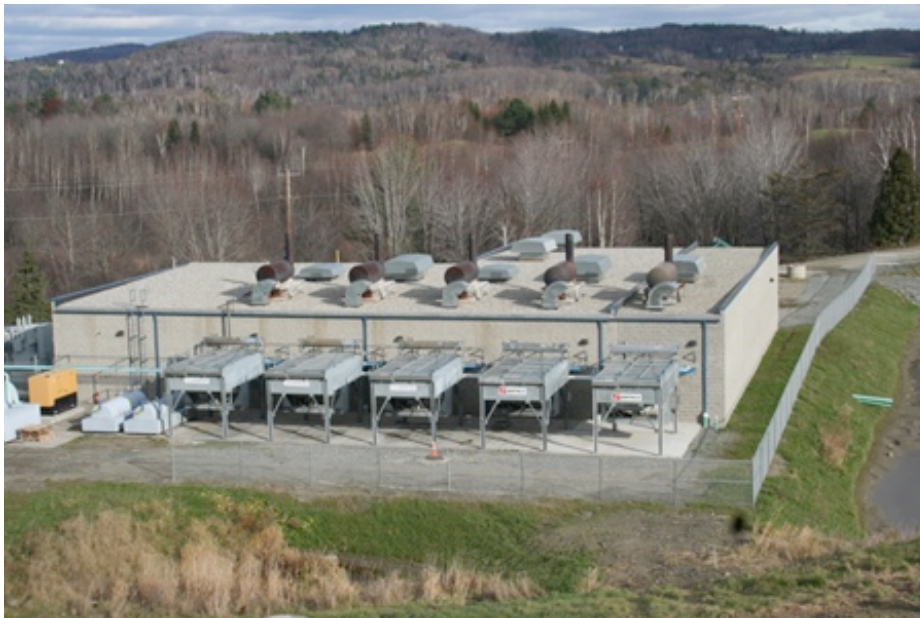
Washington Electric Co-Op's Coventry Landfill biogas plant in Northern Vermont
