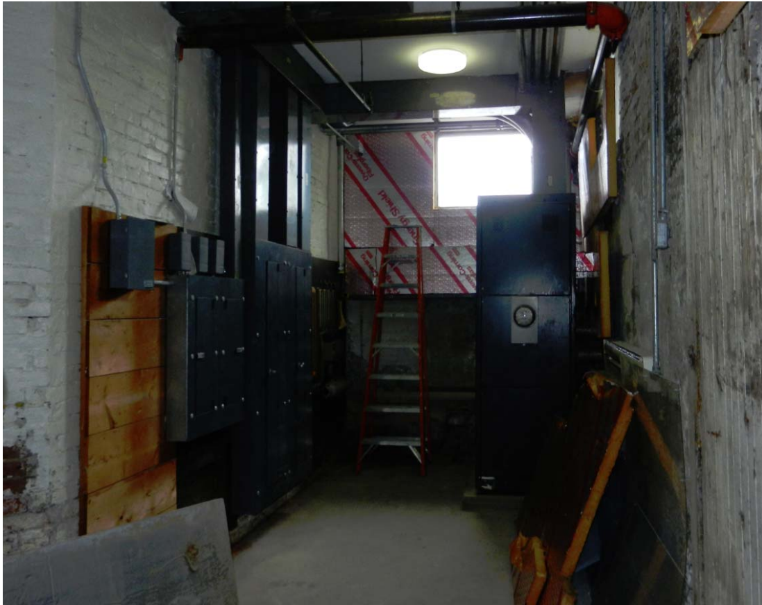
Existing Electrical area in basement
